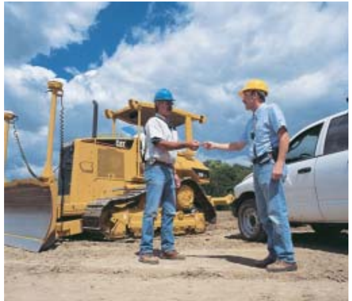
Technology training translates directly into increased productivity, whether in the office or on the jobsite.
