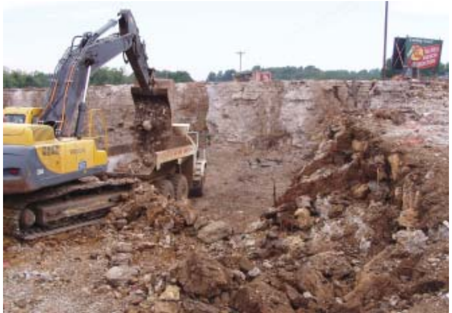
The 122-acre fast-track Crackerneck Creek retail site in Independence, Missouri, is being completed with the use of wick drains and drainable rock, precise surveying models and machine control from Leica Geosystems. The finished site will showcase an aesthetic and functional lake feature and basin.
