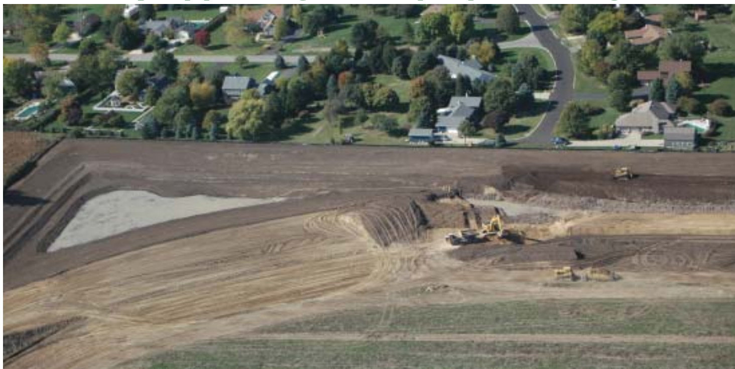
This complex basin at West Point Gardens in Elgin, Illinois, was graded and shaped with Topcon's 3D-GPS+ machine control systems. It is designed as a "wet pond" that will enhance the residential neighborhood and control stormwater.
